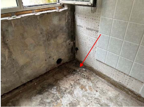
Open window to stairwell to first floor – no evidence of birds or bats noted. Scattered bird feathers and droppings to western side of first floor with larger accumulation of droppings to open window (in W/C) on western side.
