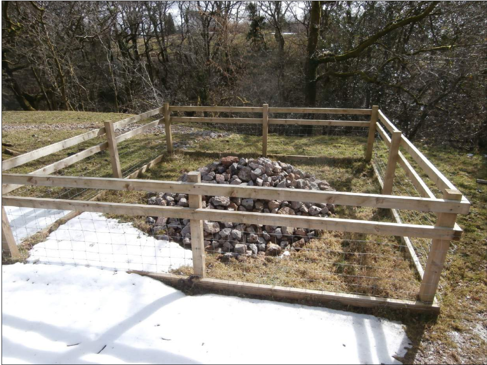
FIGURE 16 TREATED LLWYNAU MINESHAFT (C.A. 304185-011) LOOKING SOUTH WEST. TAL-Y-FEDW FARM VISIBLE ACROSS THE VALLEY OF THE NANT MYCHYDD
